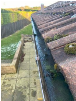
Standing water in gutter
