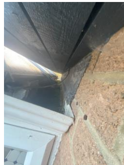
Debris in boxed gutter
