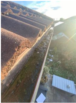
Standing water in gutter
