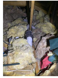
Fan ducting not insulated
