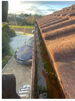
Standing water in gutter
