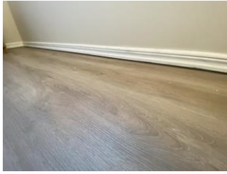
Gap between floor covering and skirting
