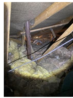
Daylight showing through eaves
