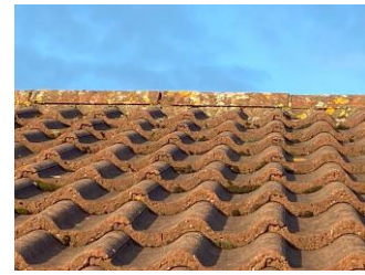
Moss on ridge tiles
