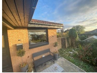
Vegetation in gutter
