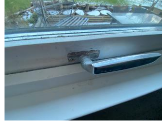
Rust/corroding window handles
