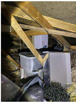
No access to boiler
