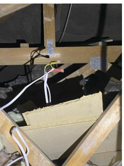
Spliced electrical connections
