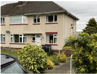
Pebble dash repairs and minor cracking
