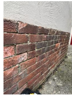
Blown brick face to stair wall
