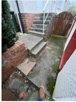
Cracked concrete pathway
