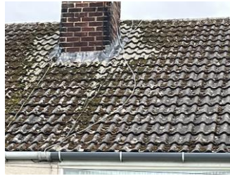
Moss around chimney stack
