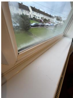
Condensation on inner pane
