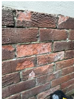
Blown brick face to stair wall
