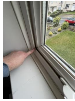
Window not locked into its housing correctly
