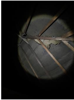
Torn/perished roof felt
