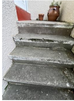
Blown concrete stairs
