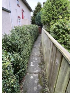
Maintenance required to fencing to prevent rot and decay
