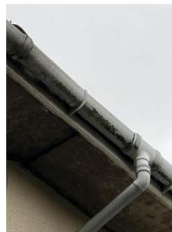
Paintwork to timber fascia
