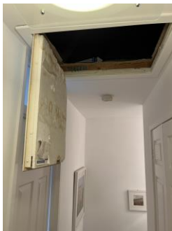
Insulated loft hatch
