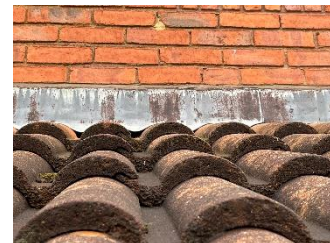
Staining of lead work
