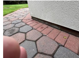
DPC could not be seen to conservatory base
