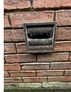
Damaged extractor grill
