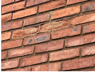
Patches of blown brick face
