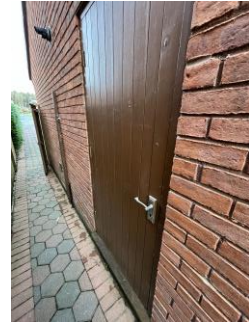
Timber door on side elevation showing decay to weather board
