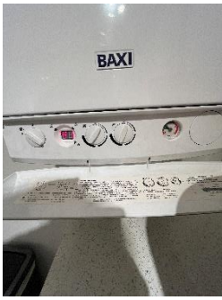
No warnings on display
