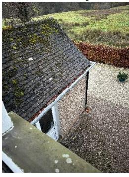
Vegetation in gutters
