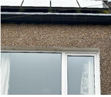
Structural cracking around lintel
