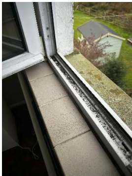
Leak to underside of window
