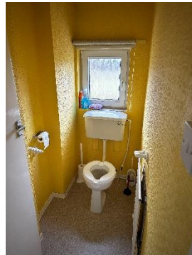
WC connect via lead waste
