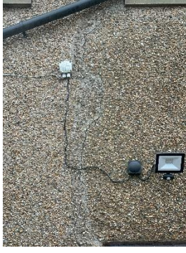
Thermal cracking of pebble dash
