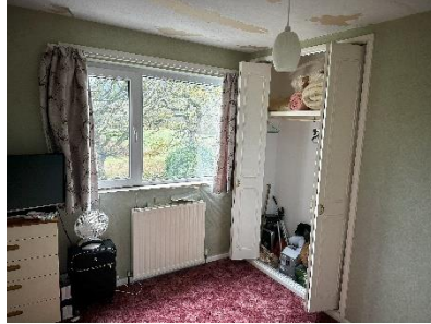
De bonded wall paper due to condensation
