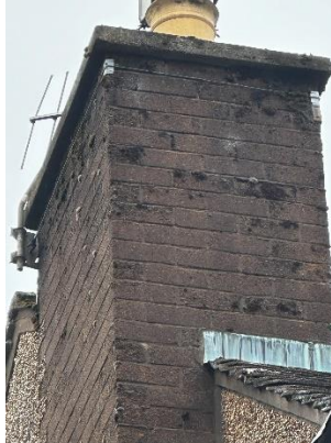
Moss on chimney stack
