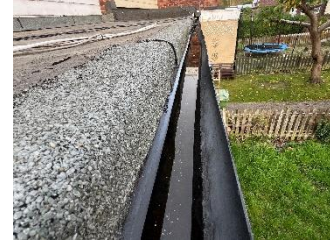
Pic3: Evidence of back falling guttering
