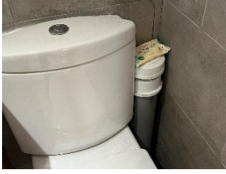
Pic4: Cistern is loose with cracked silicone
