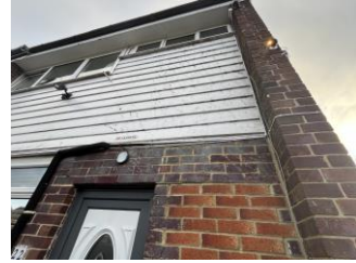
Pic3: Evidence of vegetation growth on timber cladding
