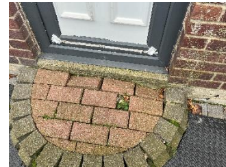
Pic3: missing weather bar
