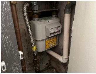
Pic1: Gas meter
