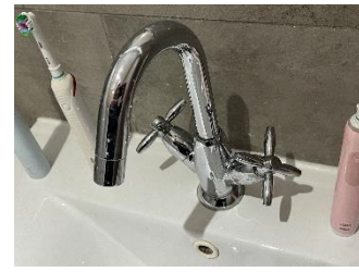
Pic3: loose sink tap
