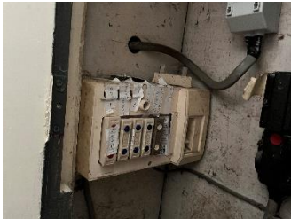
Pic1: Old fuse wire board
