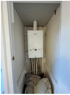
Pic1: Boiler location
