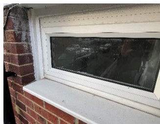
Pic5: Gap between frames
