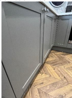
Pic2: Misaligned doors
