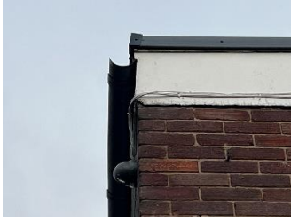
Pic1: Stop end missing from main roof gutter
