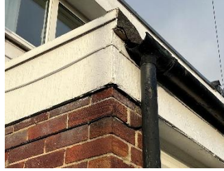
Pic2: Stop end missing from single storey roof gutter
