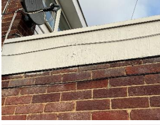
Pic1: paint flaking
