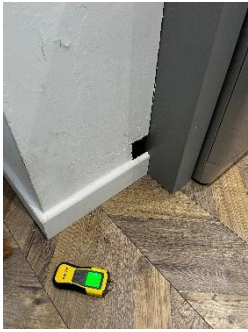
Pic1: Rear door reveal paint flaking
