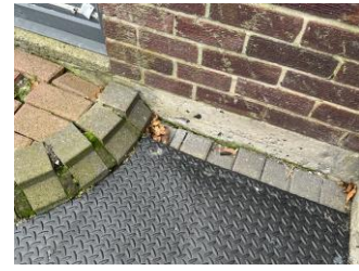
Pic3: slipped block paving
