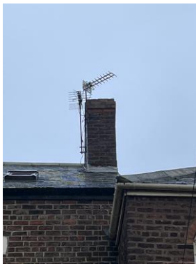
Leaning chimney stack
