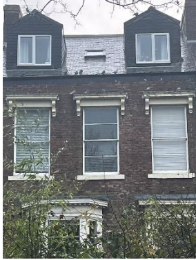
Windows appear out of square
