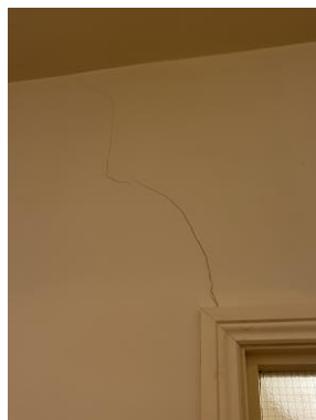
Diagonal cracking above door
