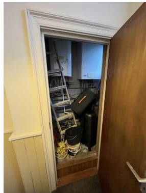
Storage in a fire risk area
