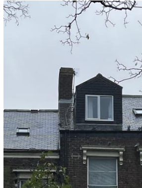
Slipped slate to left side of dormer
