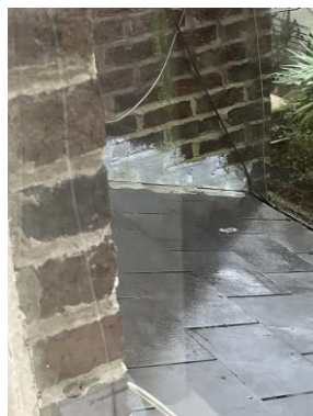
Lead upstand missing
