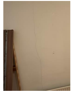
Vertical thermal cracking
