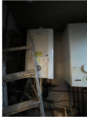
Boiler installed in service cupboard
