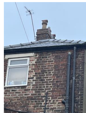
Vegetation in gutter
