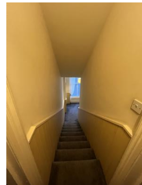
No hand holds to stair
