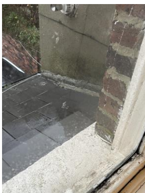
Lead upstand missing
