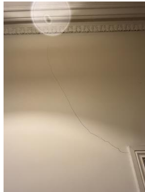
Diagonal cracking above door
