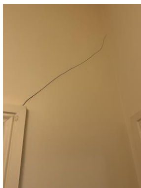
Diagonal cracking above door
