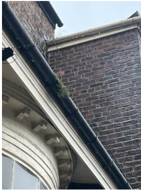
Vegetation in gutter
