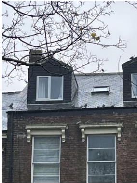
Slipped slate to left side of dormer
