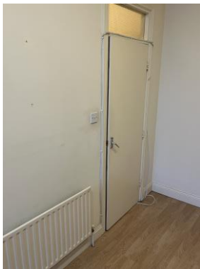
Kitchen door not latched
