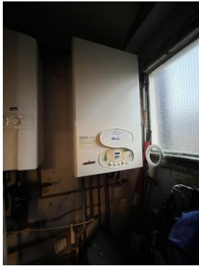
Boiler installed in service cupboard
