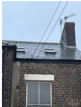
Leaning chimney stack
