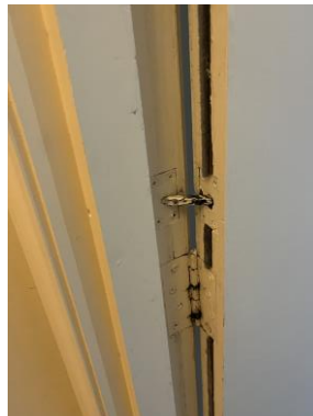
Self-closer is worn and painted
