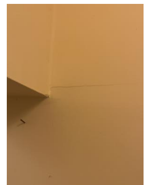
Horizontal crack near lintel
