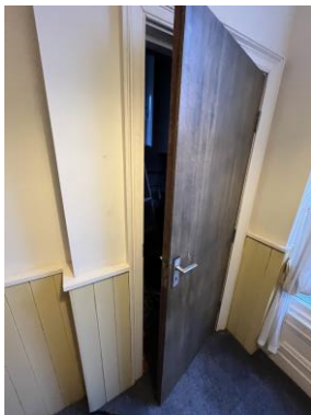
Boiler cupboard left open
