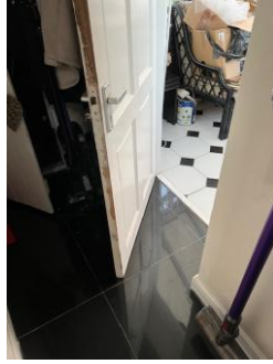
Pic 55: Door poor fitting
