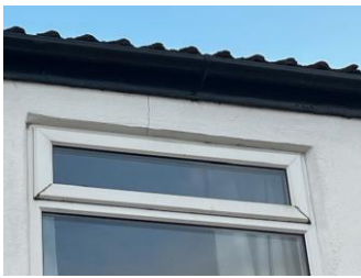
Pic 19: structural crack above window
