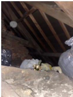
Pic 38: Reduced insulation
