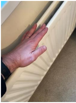
Pic 63: Bedroom radiator
