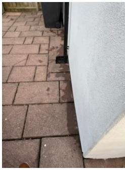
Pic 16: pathway water stained
