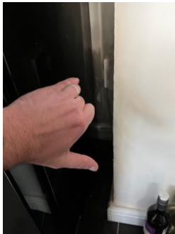
Pic 62: Stop tap behind fridge
