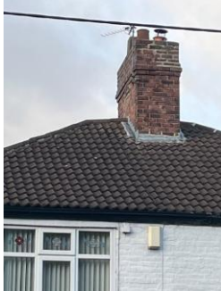
Pic 13: Ridge Deflection
