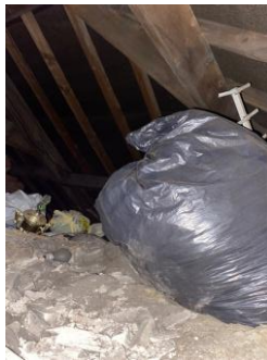
Pic 39: Displaced insulation
