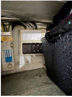
Pic 61: Fuse board
