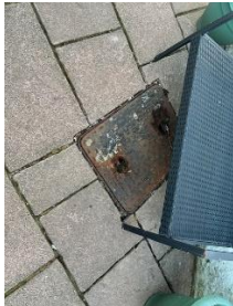
Pic 65: Drain cover
