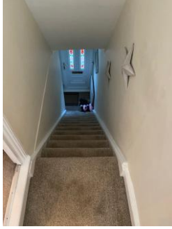
Pic 54: Missing handrail
