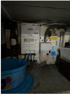
Pic 60: Electric meter
