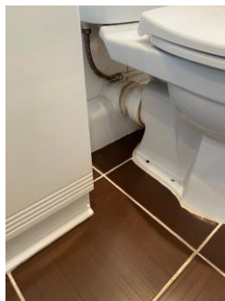
Pic 58: WC waste
