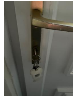
Pic 27: Operational front door mechanism
