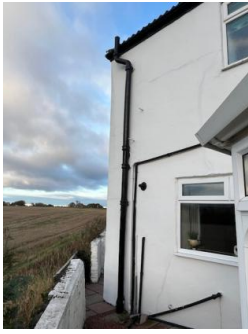
Pic 33: Missing cowl
