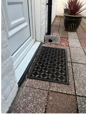
Pic : Low upstand at front door
