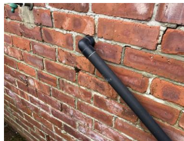
Structural crack extends across 16 courses
