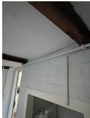
Damage to ceiling
