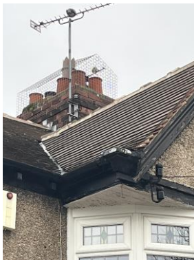
Saddle flashing not visible
