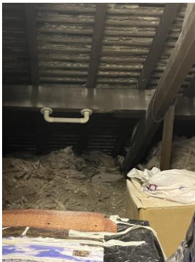
Displaced insulation blocking ventilation
