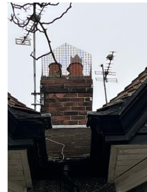
Missing pointing on chimney stack face
