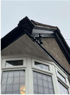
Blistering Fascia boards
