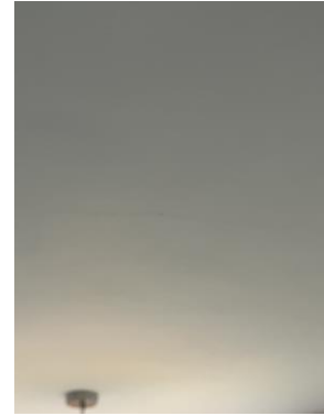
Rear bedroom ceiling
