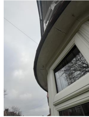
Blistering soffit boards
