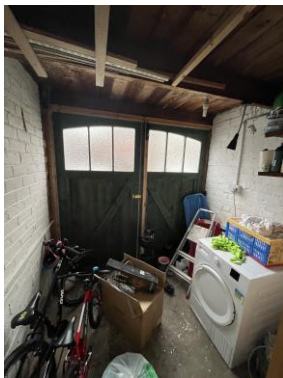
Evidence of water damage
