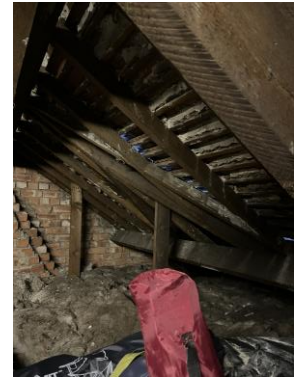
Visible daylight between tiles
