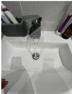
Bathroom hot water tap
