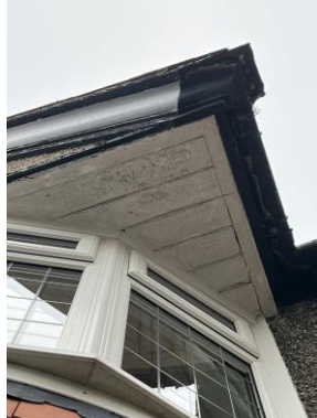
Blistering soffit boards
