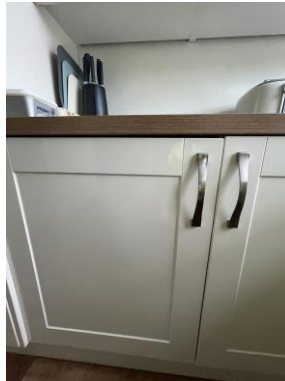
Doors need realigning
