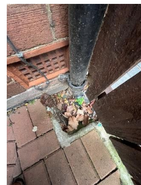
Discharge into gully
