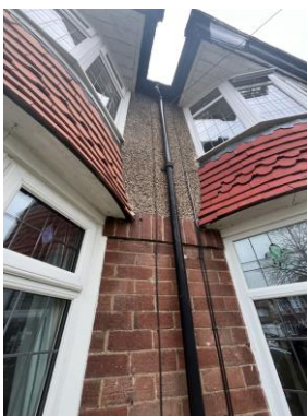
Cast iron downspout
