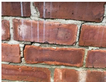
Stepped structural crack
