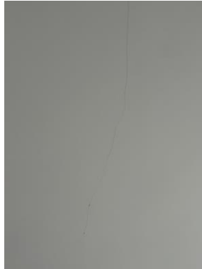
Rear bedroom ceiling
