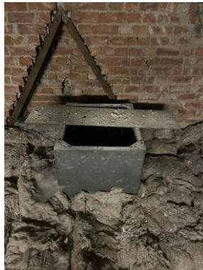
Redundant water tank
