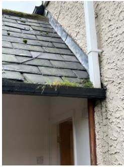
Vegetation in guttering
