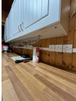
Extensive electrical extension
