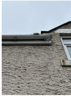
Vegetation in guttering
