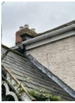
Moss and algae on roof
