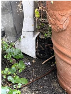
No Gully to down spout
