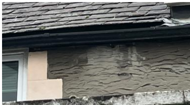
Water staining to render
