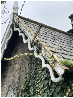
Decaying roof timbers
