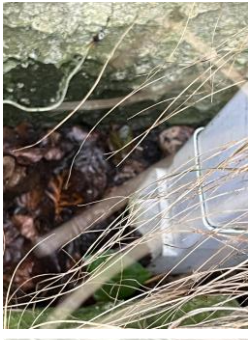
No Gully to down spout
