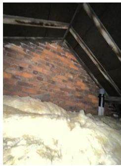
Staining to timbers
